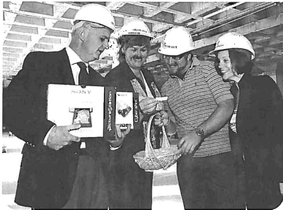
Faculty and staff campaign co-chairs Greg Finn and Karen McAllister-Kenny are joined by James O'Brien and Kim Meade as they draw the winner in the Campus Campaign participation draw in the Learning Commons construction zone. Absent is co-chair Kithio Mwanzia. Sandra Grusso, Office of International Recruitment, was the winner.
