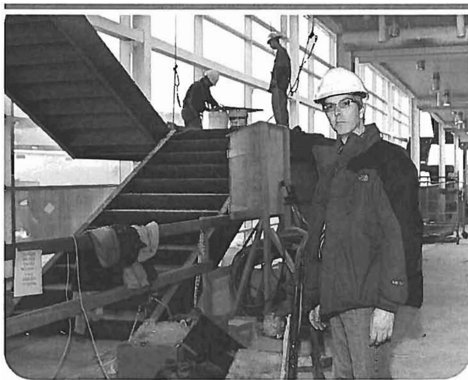
Scott Walker, Facilities Management, stands in the new Plaza2006 building last week.
