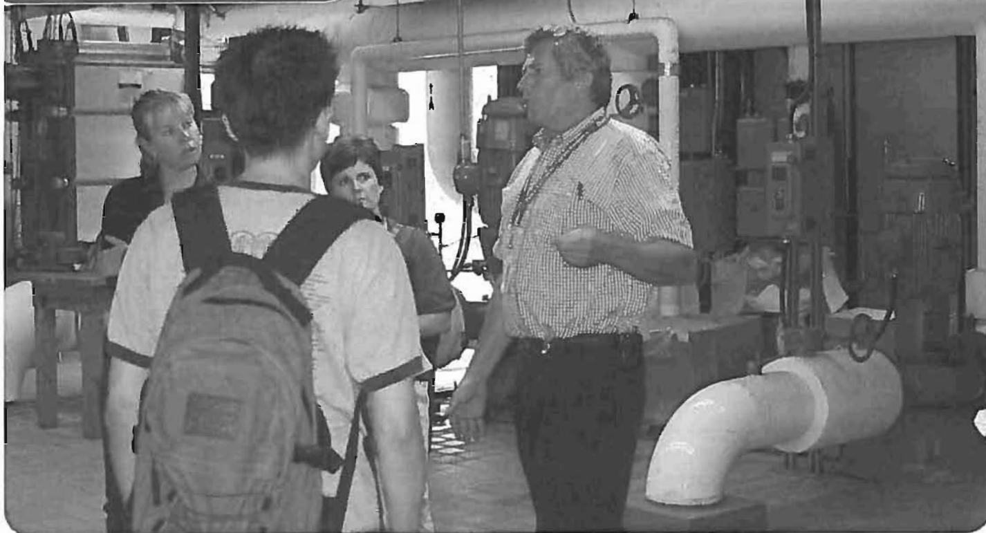
Doug Beckett, right, Manager, Maintenance and Operations, Facilities Management, takes new faculty and staff on a tour of the Cogeneration Plant as part of the recent New Faculty and Staff Orientation program held on campus Aug. 13 to 15. The orientation included several sessions over three days, culminating Aug. 15 with the Brock Family Picnic and a nature walk.
