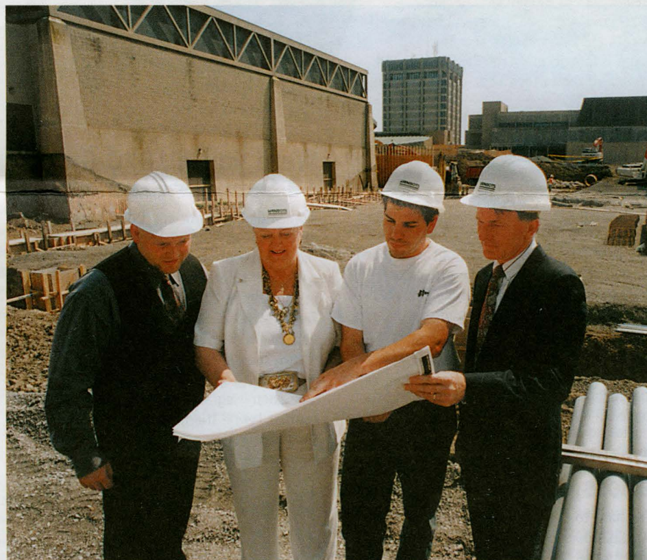
Outside the Physical Education complex, Bill Chenard, second from right, project coordinator for Vanbots Construction Corporation, points to the site plans as he explains the work under way to, from left, Rob Gilmour, Val Fleming, and Robert Kerr.
