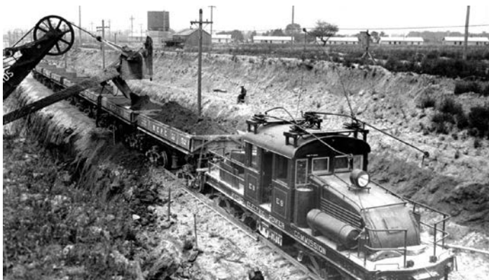
Electric locomotive c. 1918 during the construction of Sir Adam Beck G.S. #1. Courtesy Niagara Railway Museum.
