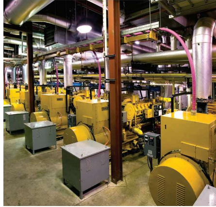
Brock University is upgrading its co-generation facility, a reliable and energy-efficient source of electricity, cooling and heating on campus.
